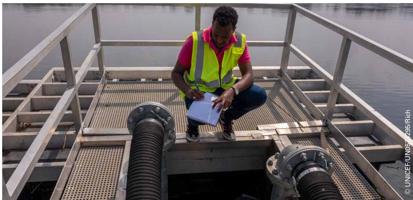
A worker monitors the Nile River water intake plant, a component of a new UNICEF-supported water purification and pumping system serving residents and internally displaced persons in Juba, South Sudan.
