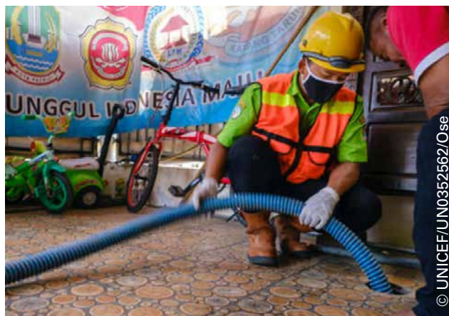
A worker from the Bekasi Sanitation Department, near Jakarta, Indonesia, empties the septic tank of a local resident for transport to a safe waste water management site.
