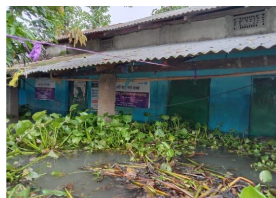
UNICEF-supported learning center got damaged in Sunamganj district
