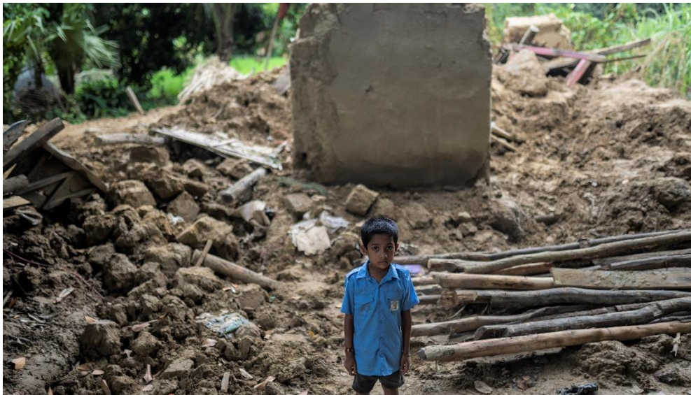
Little Ovi stands forlornly next to the ruins of their house as a result of damage caused by a landslide in Lama, Bandarban in August 2023. Left with nothing, he and his family have sought refuge in a relative's house. In the face of such climate emergencies, UNICEF remains dedicated, working tirelessly to provide essential services such as water and sanitation, healthcare, and protection, striving to rebuild shattered lives in the aftermath of this natural disaster. © UNICEF Bangladesh/2023/Mukut
